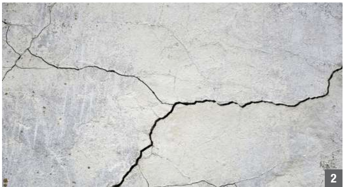
Presence of cracks
