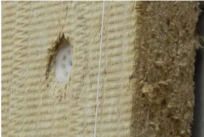
Example of an incorrectly installed anchor
