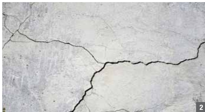
Presence of cracks
