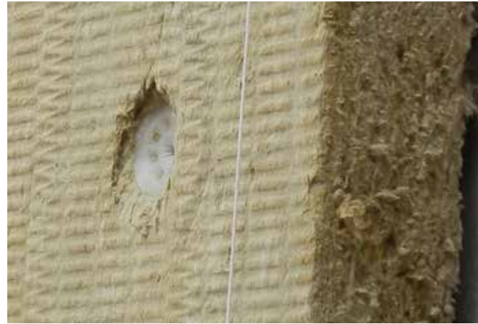
Example of an incorrectly installed anchor
